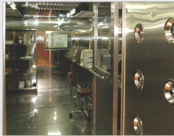
Clean Room System
