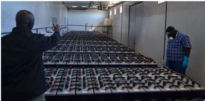
Battery storage facility at the Tsumkwe plant in Namibia.
