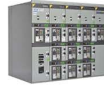
Power distribution and circuit protection
