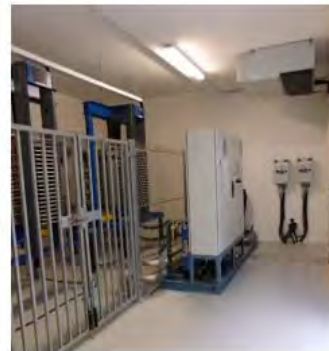
Thyristor valves room
