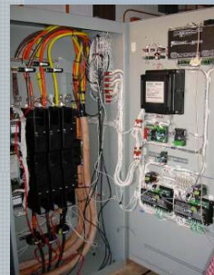
Switchgear, Relays, & Controls
